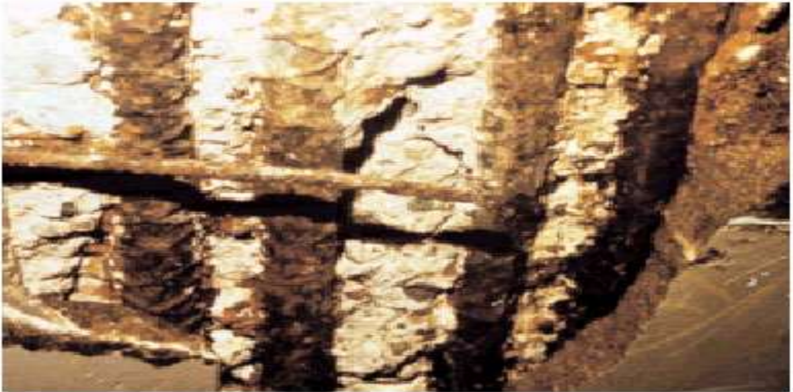
Fig. 6-16. The damage to this concrete parking structure resulted from chloride-induced corrosion of steel reinforcement. (50051)
